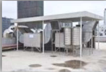
Paint Shop Ventilation
