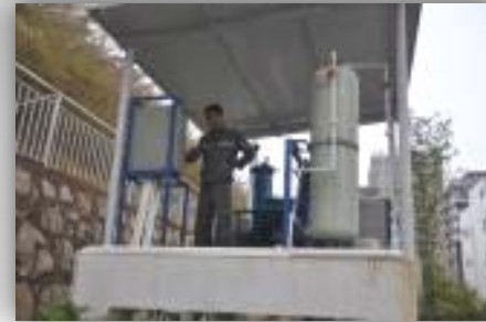
Car Wash Water Recycling
