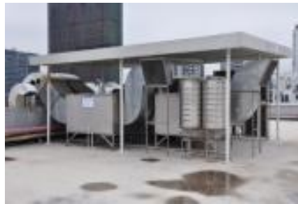
Paint Shop Ventilation
