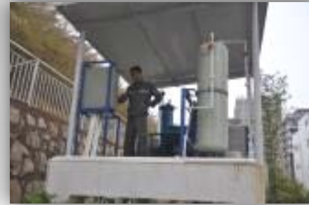
Car Wash Water Recycling
